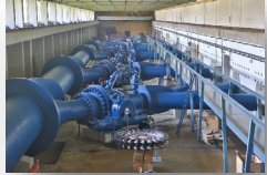
Machine room at Lünseewerk, since 1970
