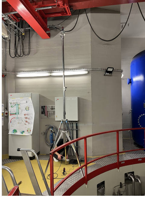
Figure 3.2: Hydropower Plant Rodundwerk II.
