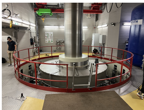
Figure 1.1: Hydropower Plant Rodundwerk II
