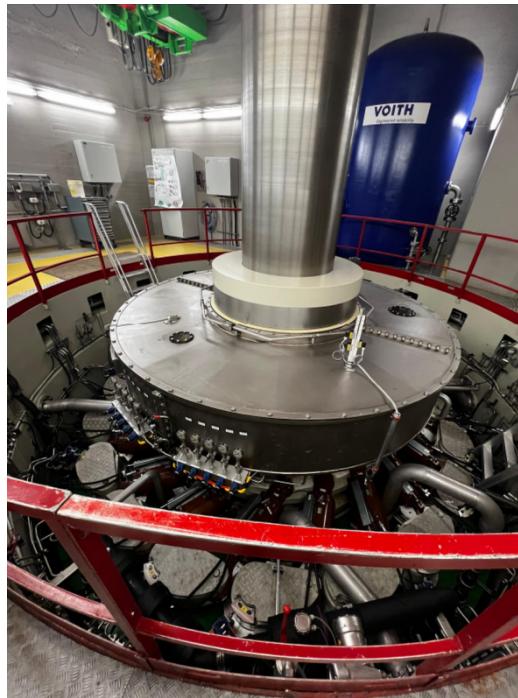
Figure 1.1: Machine Room Rodundwerk 2 [5]
